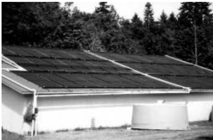
Solar water heating at the Rosewall Creek salmon hatchery on Vancouver Island, BC. (Photo courtesy Taylor Munro Energy Systems)
