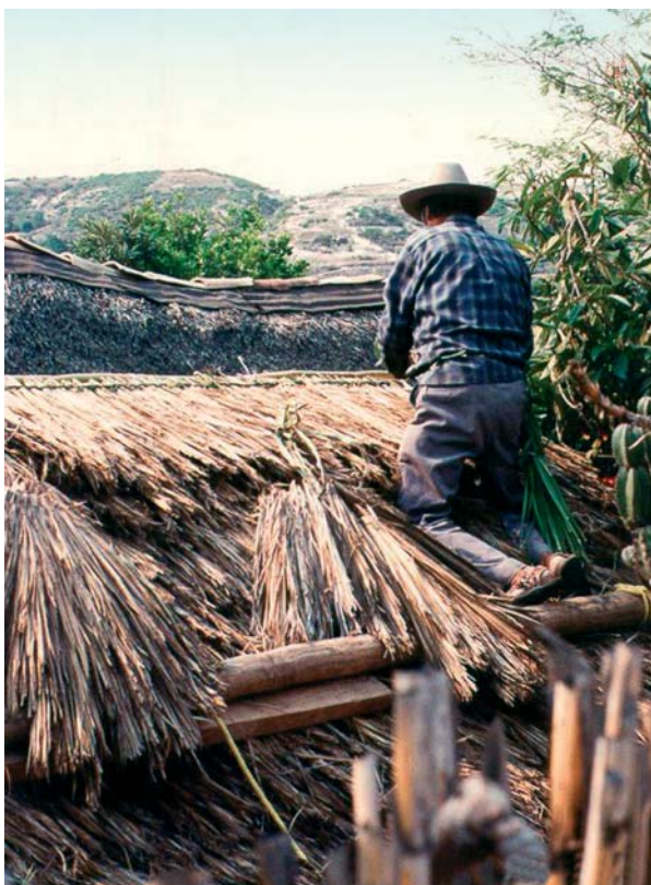
Re-thatching a roof with the versatile soyate palm in the community of Topiltepec, Guerrero, Mexico.
